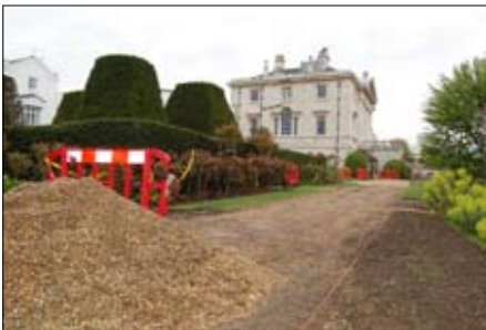
Base, a combination of compacted coxwell self-binding gravel and old gravel on MOT.
