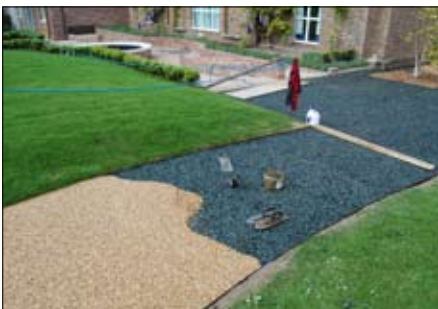
Applying the aggregate resin bound top coat mixture to the easylay™ rubber sub-base
